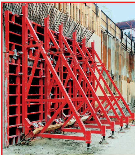
SB-B and SB-C brace frame units with PERI TRIO panel formwork, concreting height 3.50m.
